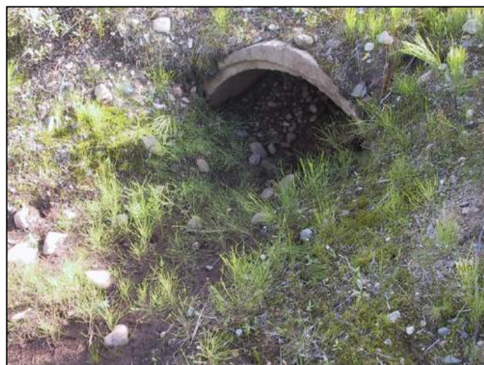
Figure 8.3: Blocked pipe culvert that requires cleaning
